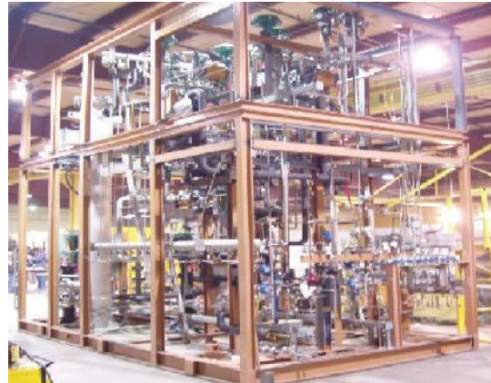
Engineered Module Tritium Removal Facility Dryer Skid
